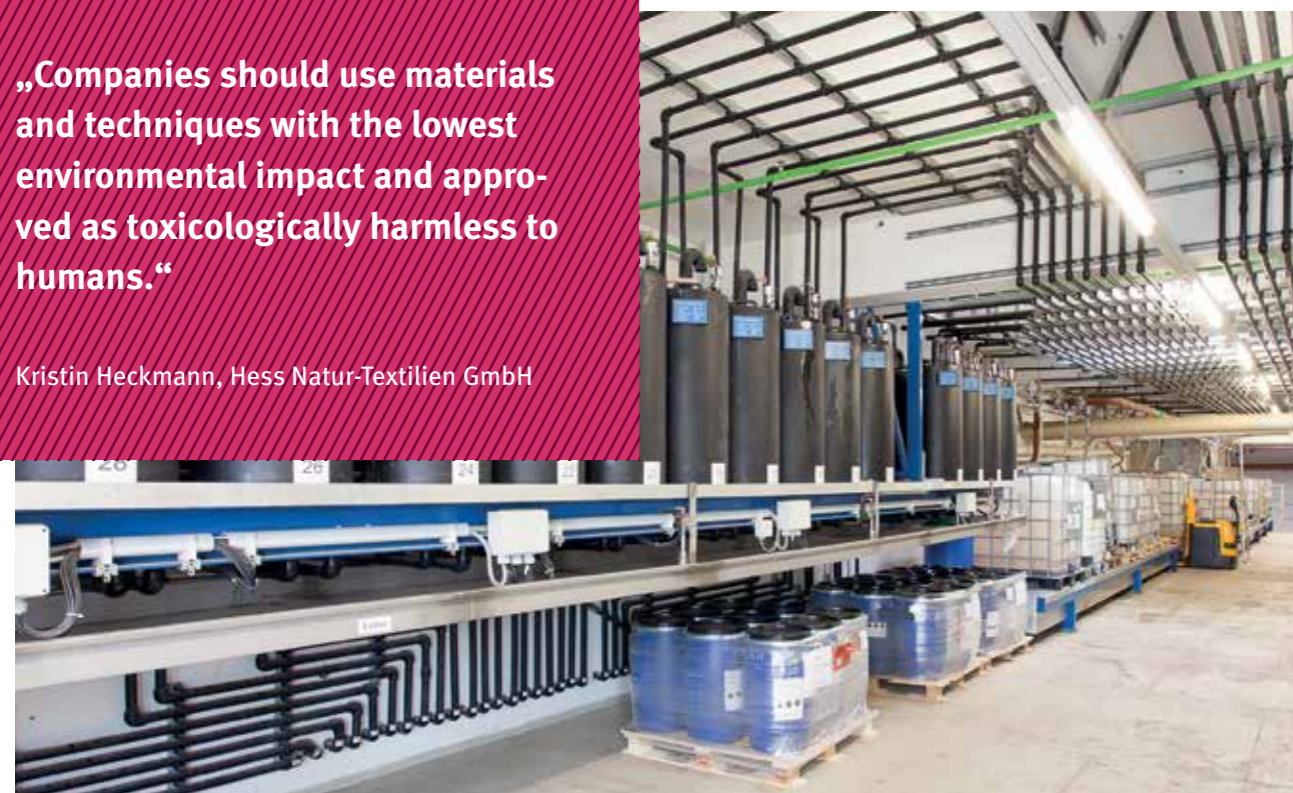
Optimized transfer of chemicals from storage to the batching tanks. The tanks are directly connected with the chassis.
